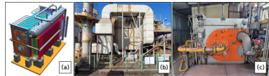
Fig. 1. Mixed gas boiler, (a)Boiler body, (b)Gas duct, (c)Burner set.
